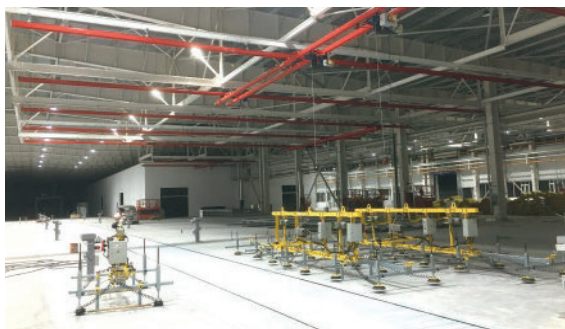
Electric Walking - Electric Lifting (Double Beam KBK)(500KG)
